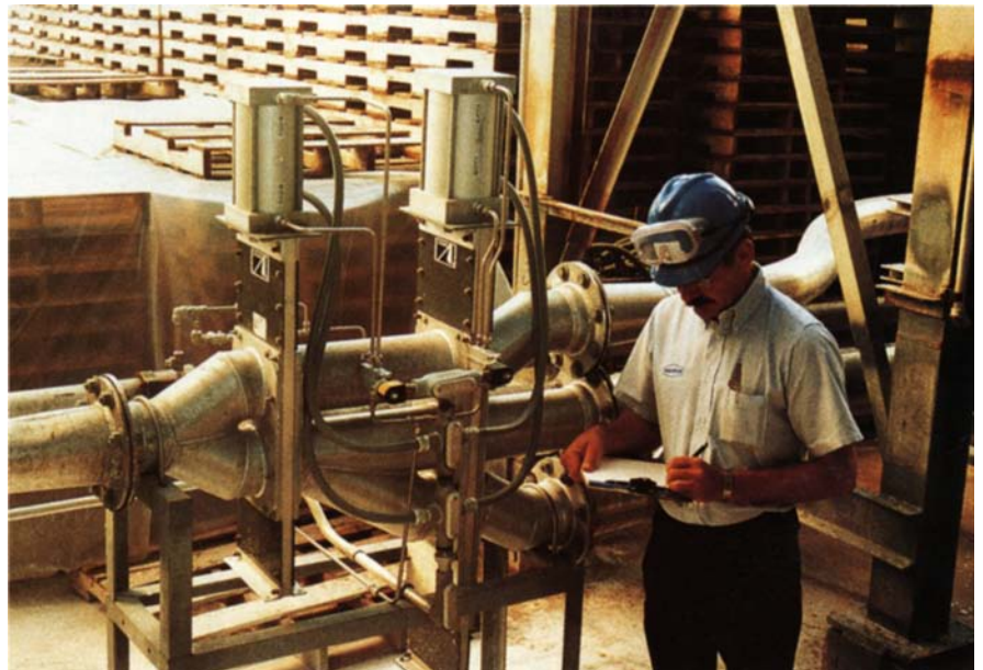
Melamine powder is routed from storage to filling and packaging by diverter valves. Ray Duet inspects a vertically mounted, three-way valve.
