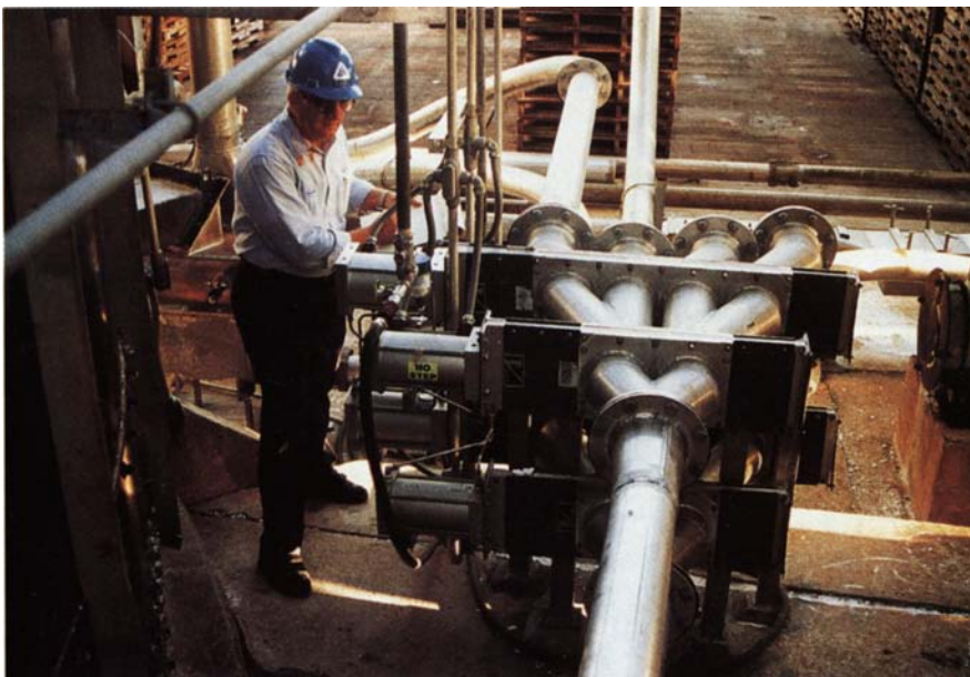
The chemical plant installed many four-, three-, and two-way diverter valves. Carl Schroeder is shown with a horizontally mounted, four-way unit.
