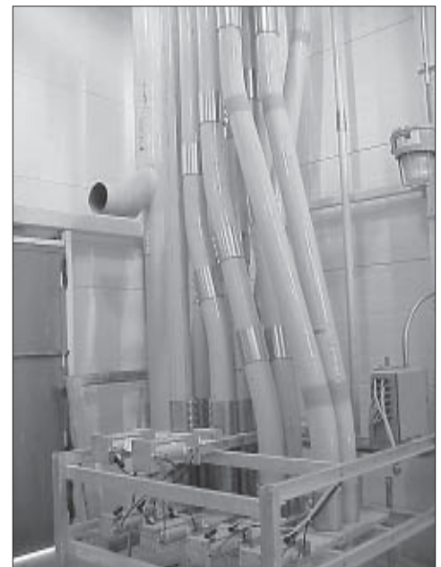
Valve station 1 distributes flour to valve station 2 or to storage bins using 6-inch-diameter lines.
